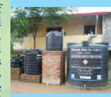
Rain water Harvesting Unit
